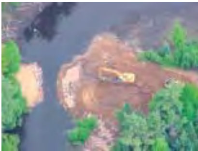
Thursday morning 6/7/01. Following drawdown, breaching, and channel relocation on the first two days, the contractor is preparing to widen the new channel to match the natural river width.
