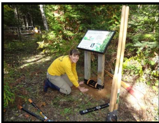
Photo: Installation of a new boot brush to prevent the spread of invasive species at the North Bay State Natural Area in September.
