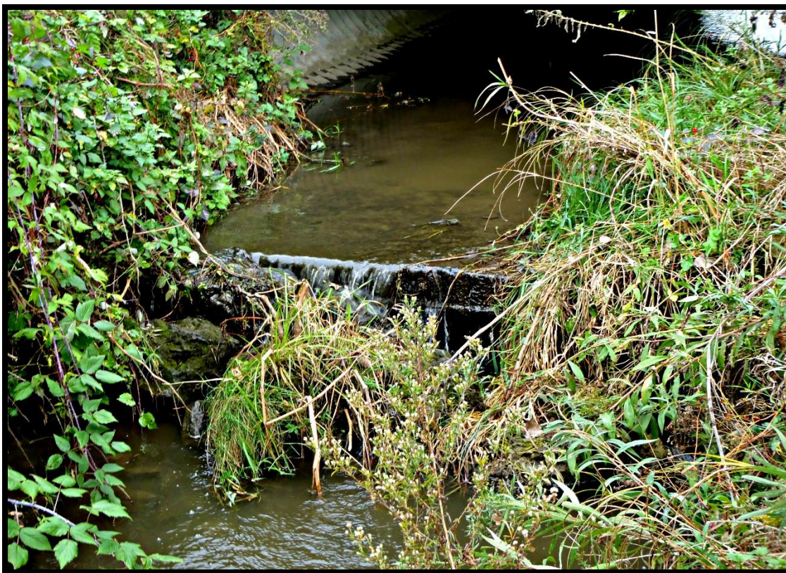
Unnamed Stream, WBIC 929400, at CTH E illustrates a perched culvert. Photo by James Amrhein, Wisconsin DNR.
