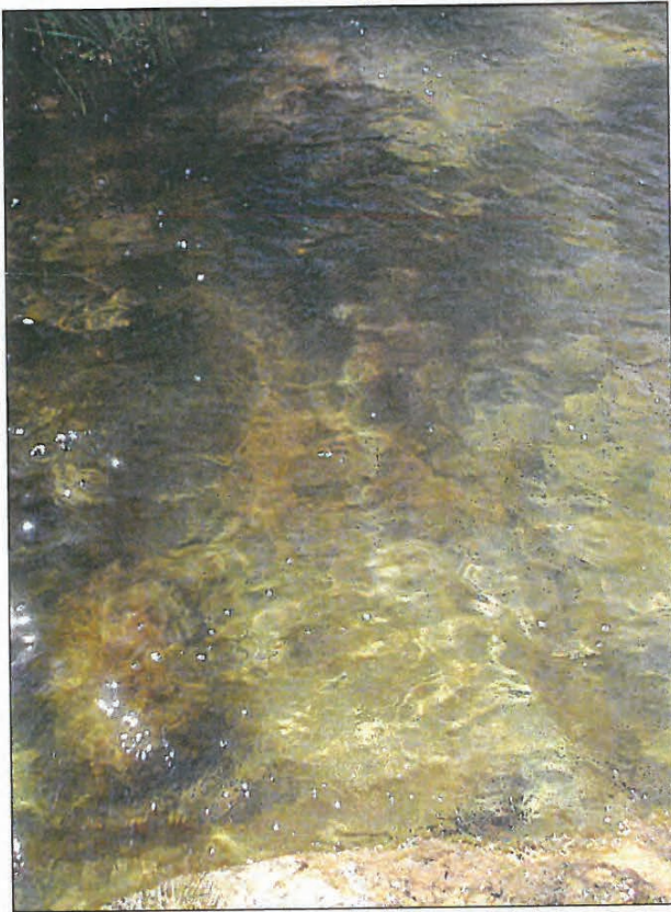
Photo #10 – Hooker Lake Dam (deteriorated spillway) (May 20, 2009)
