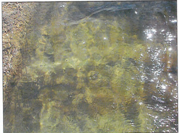
Photo #11 – Hooker Lake Dam (deteriorated spillway) (May 20, 2009)
