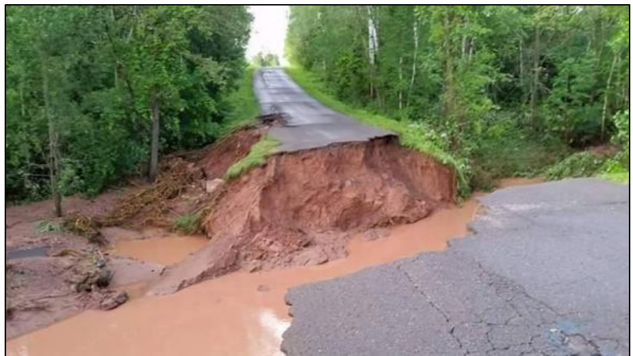
Road damage in Bayfield County after July 2016 flood event. Photo courtesy of Bayfield County.
