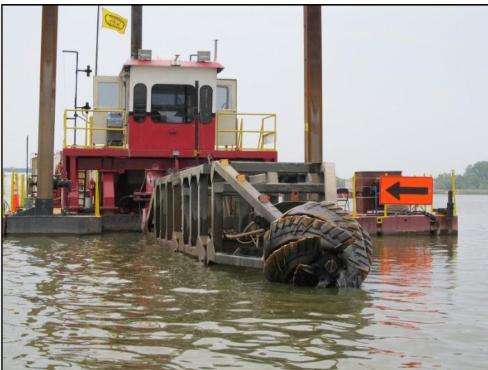
Pictured above is the hydraulic dredge that is used to remove sediment from the Fox River. The cutter head spins at the end of the arm, which pulls sediment into large pipelines that then transport the sediment to a facility offsite for processing and treatment. Photo by: Cheryl Bougie, DNR.
