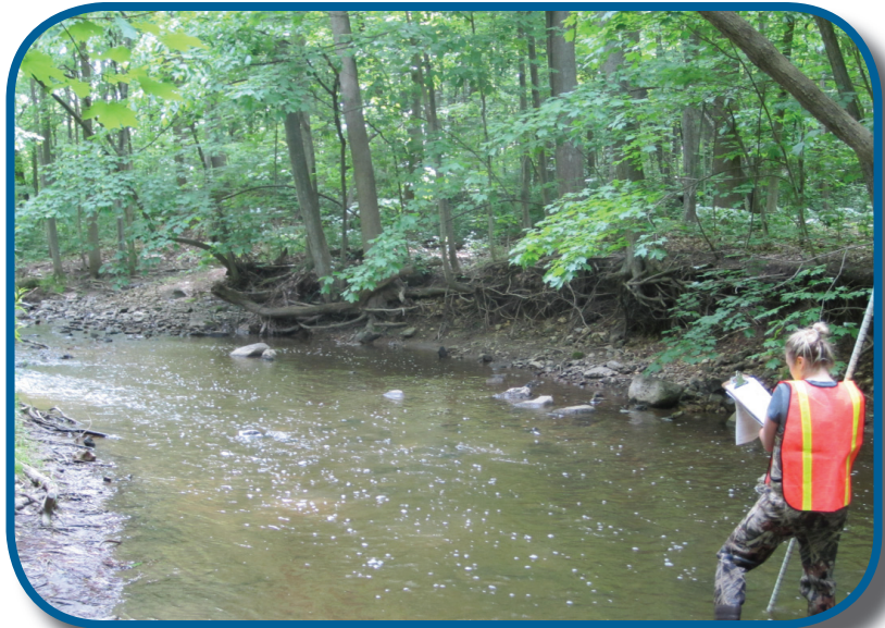
Erosion is evident in this portion of Hoods Creek.
