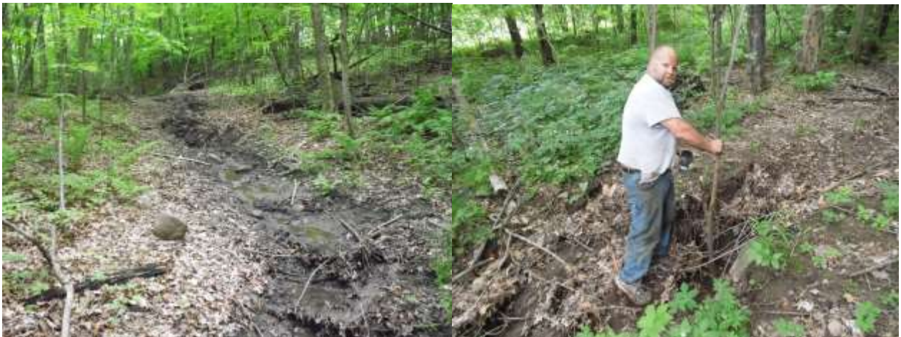
Figure 17 – Washout between the top of the 53 & V field and Bear Creek in June 2016 (Blumer, 2016)
