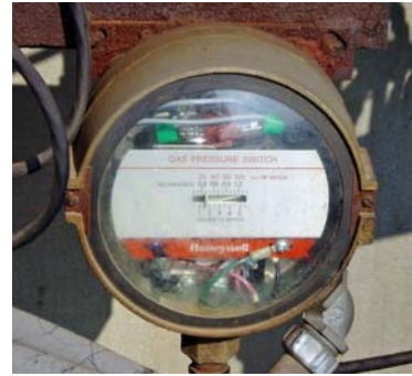
Figure 13 Mercury-containing industrial switch
