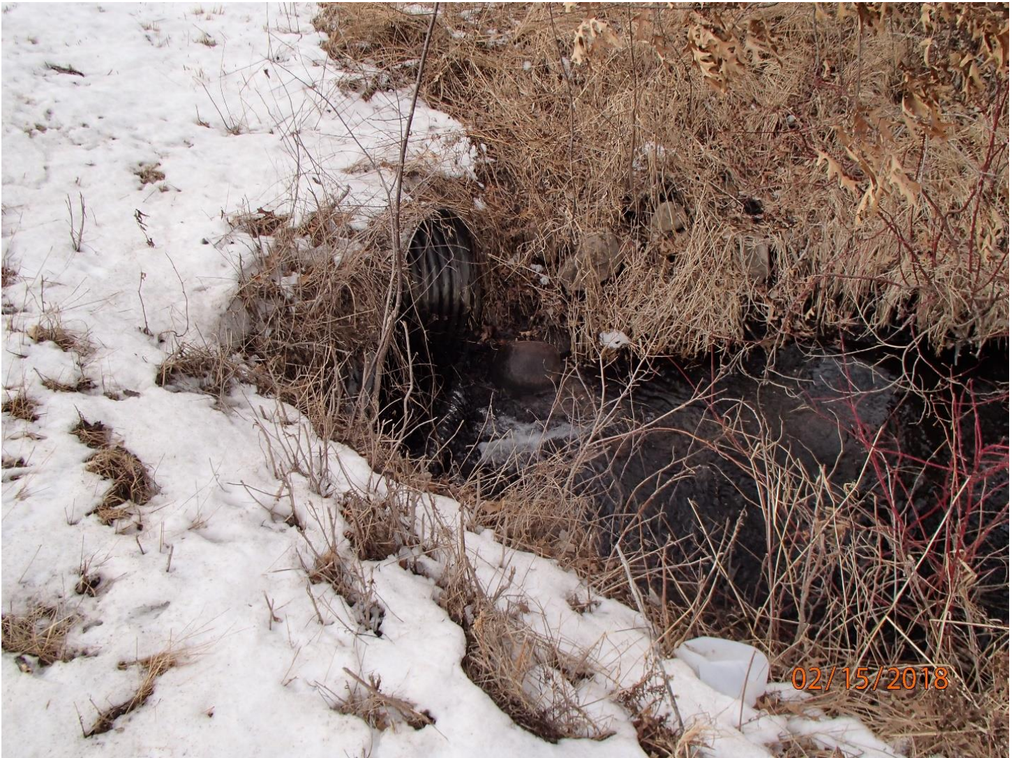
Photo 9: Perched Culvert on Kaminski Creek at County A. Photo taken by D. Bolha on February 15 th , 2018.
