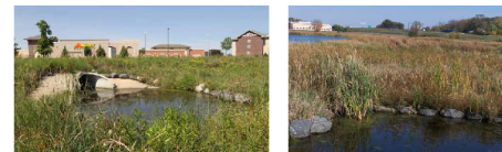
Storm-water outlet near T. domingensis colony near Esser Pond. Typha domingensis colony near Esser Pond.
