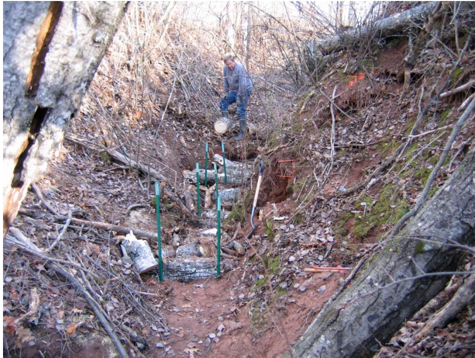
Figure 12. Roughness elements (anchored wood) installed in upland gullies draining to the Bark River. Photo courtesy of Faith Fitzpatrick.
