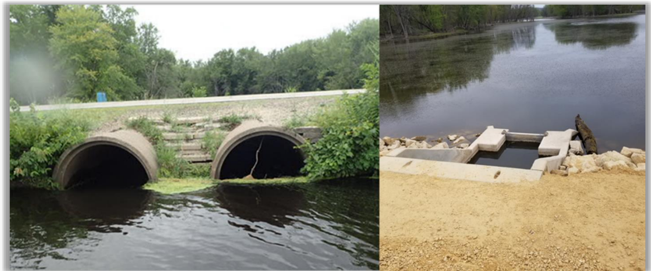
Climate change infrastructure adaptation example. Photo on left shows pre-project uncontrolled culverts. Photo on right shows post-project water control via stoplogs up to river elevation of 632 feet. At water surface elevation greater than 632 feet, water is uncontrolled. This adaptation was effective in controlling the high volume of cold water during high discharge winters that was negatively impacting winter fish habitat in this backwater of the Mississippi.
