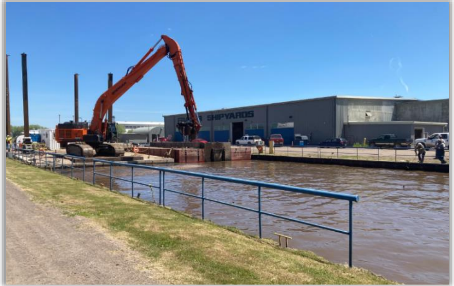
Dredging at Howards Bay, in the St. Louis River AOC. Photo by Fraser Shipyards.
