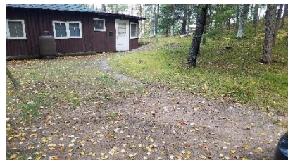
Photo 26: Sep 21, 2019. Runoff from the driveway runs around the house and towards the lake.
