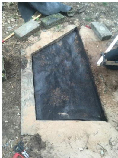
Photo 20: June 9, 2020. Filter fabric folded over top of pit. Rock layer will be added on top.
