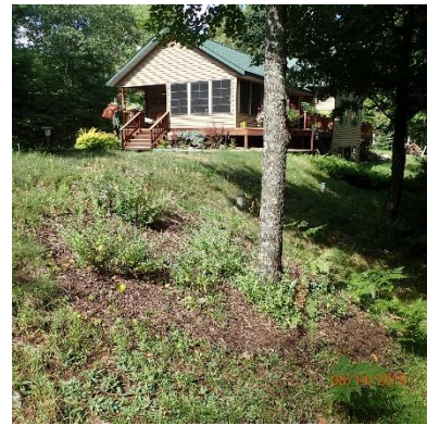
Photo 32: Aug 14, 2019. There is some erosion on the slope face near the lake.
