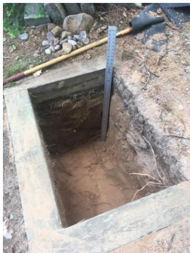
Photo 18: June 9, 2020. The owner dug 3 ft. deep holes for the infiltration pit in the steps.
