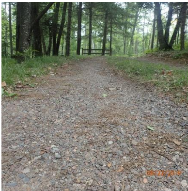
Photo 25: Aug 22, 2019. Some erosion on driveway is evident.
