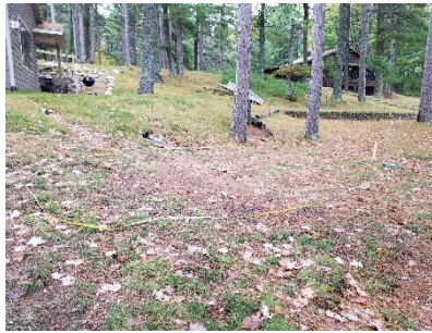
Photo 2: Oct 4, 2019. Gutters directed roof runoff and was creating some erosion issues.
