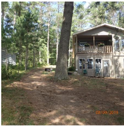
Photo 1: Aug 9, 2019. Driveway around home had ruts from use and erosion.
