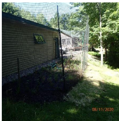
Photo 33: Aug 11, 2020. A rain garden and deer fencing were installed to manage stormwater from the garage.
