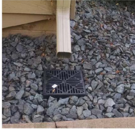
Installed collection box
