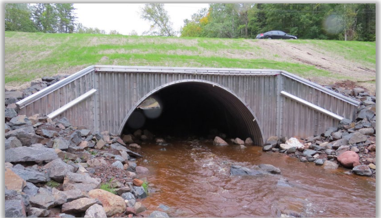
Replacement culvert for improved fish passage and flood water conveyance at Little Balsam Creek.
