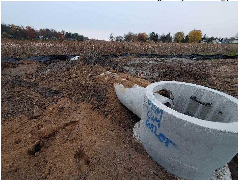
Figure 1. IESF outlet installation, October 28, 2023
