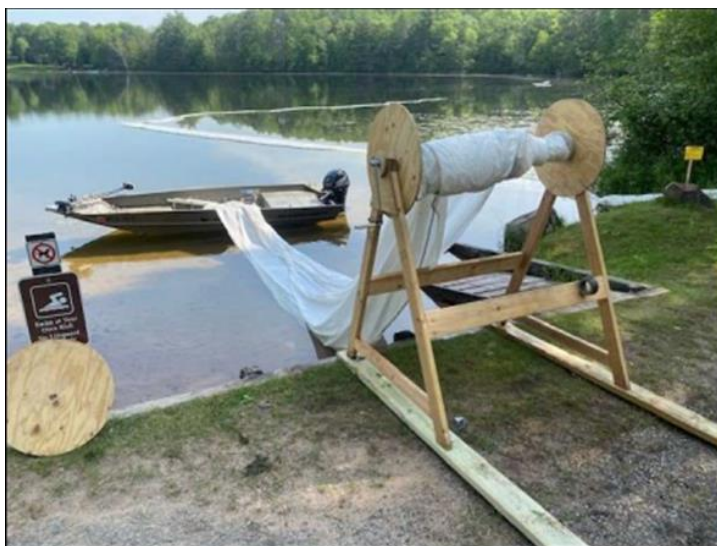
Figure 52: Limno-curtain material on a roll before installation (photo from Marinette Co. LWCD)
