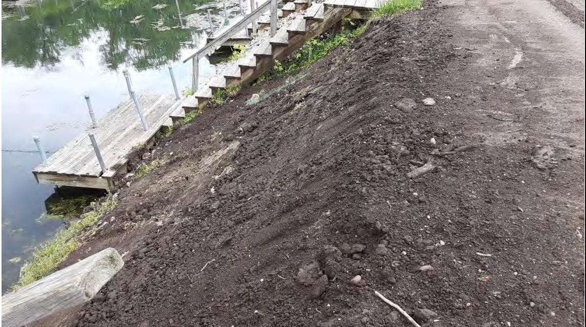
Apparent topsoil placement with no perimeter control or cover
