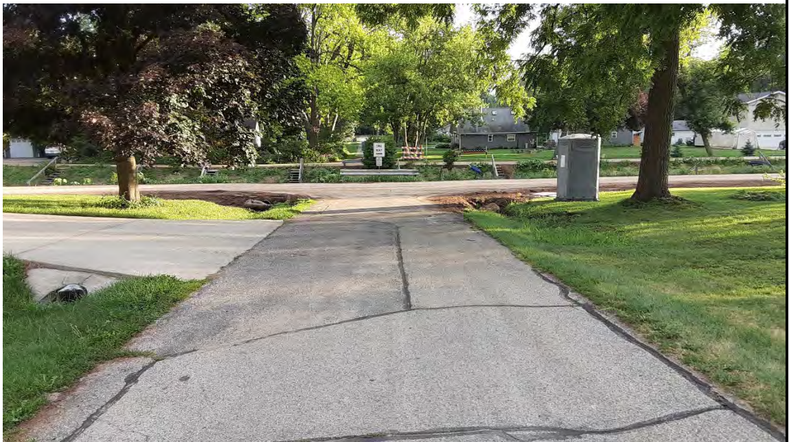
Culverts at Mulberry and S Channel Drive. SESC measures need to be maintained to ensure culverts do not clog. Current measures are not secured.
