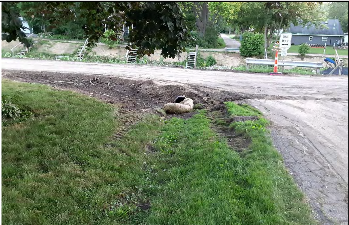
Replaced pipe section beneath South Channel Drive. SESC measures need addressing. See comment C on Site Inspection 7/11, 7/12
