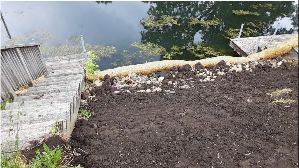
Placed perimeter control atop stone and improperly staked
