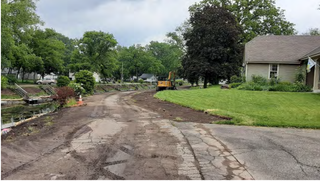
North Channel Drive – sediment tracking on roads
