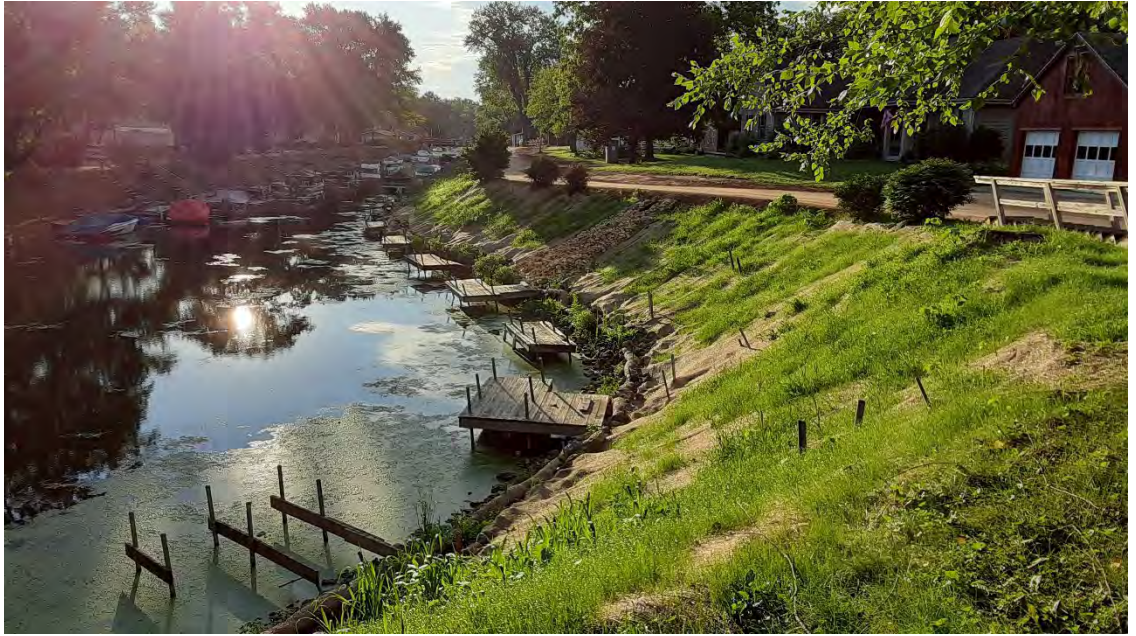
Closeup of a reinforced section, continue to monitor vegetation
