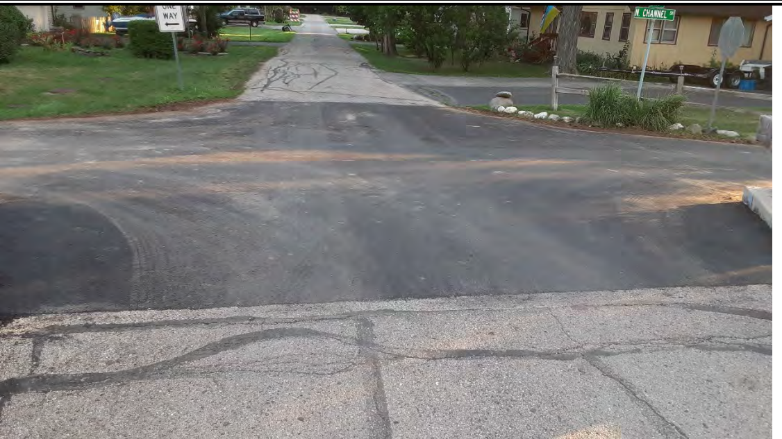
Road paving completed, typical connection at N Channel Drive and bridge at Central Blvd
