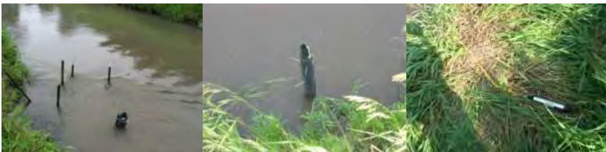
Figure 11 – Installation of pressure transducers (data logger) to measure depth of water (Papanicolaou, 2017)
