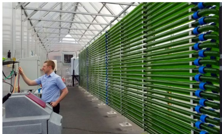
Applied Technologies Inc. staff evaluate the photobioreactor's operating conditions inside the greenhouse which contains the ABNR system.
