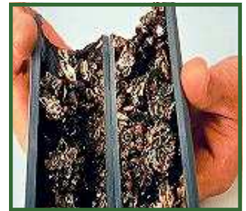
zebra mussels in a intake pipe
