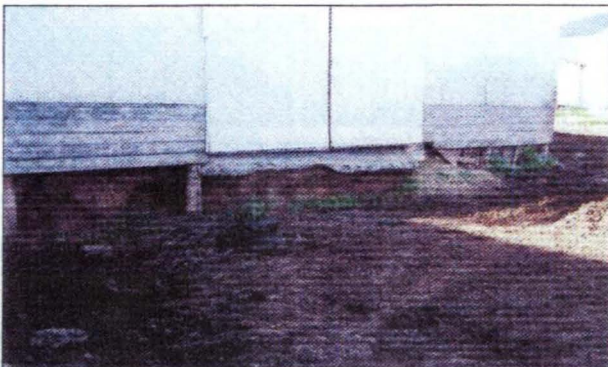
Before: Just prior to construction, the barnyard shows a destabilized building foundation.
