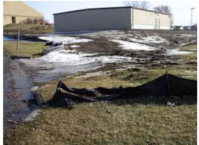
Construction Site Erosion, Dunn County. DNR Photo.
