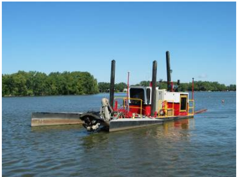
A hydraulic dredge used on the Fox River, Wisconsin in 2006 to remove contaminated sediment.
