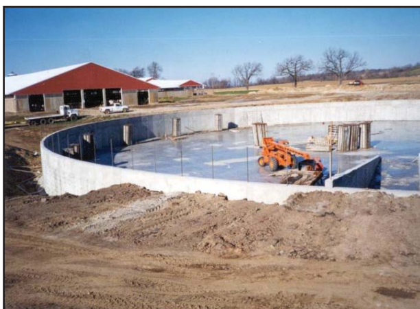
Construction of concrete manure storage facility at a CAFO Photo Courtesy of WDNR
