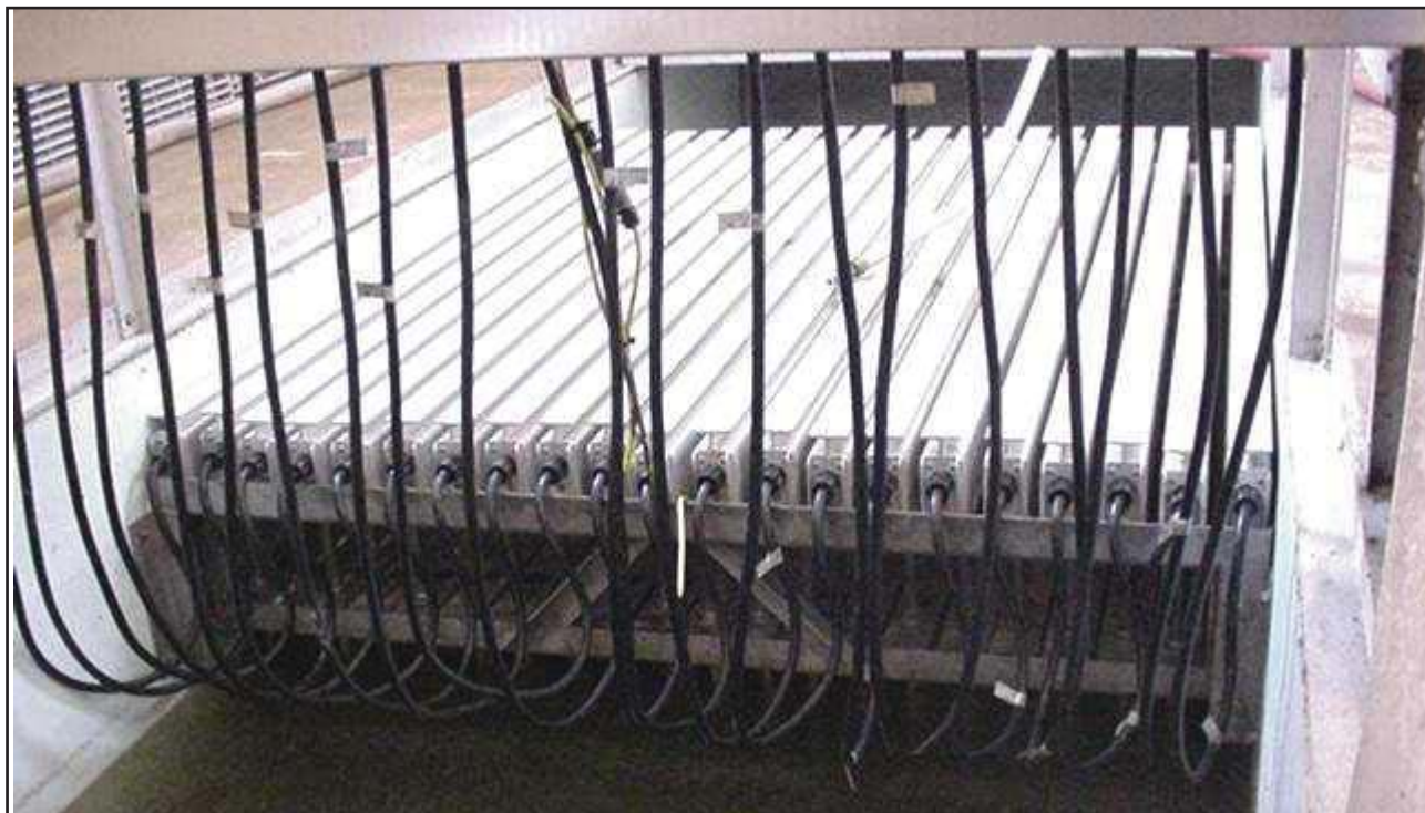
Ultraviolet Radiation Wastewater Treatment Plant System, Photo Courtesy of Julia Riley, WDNR
