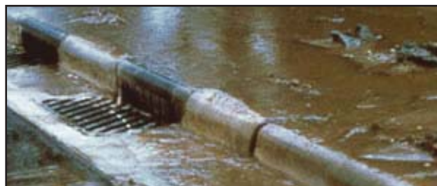
Construction site erosion running into a storm drain that eventually makes its way to a local stream or lake. Photo Courtesy of WDNR
