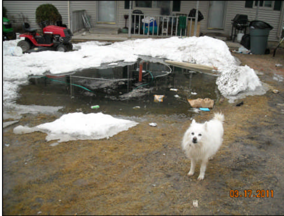
Before – A failing holding tank discharging effluent to the ground surface.
