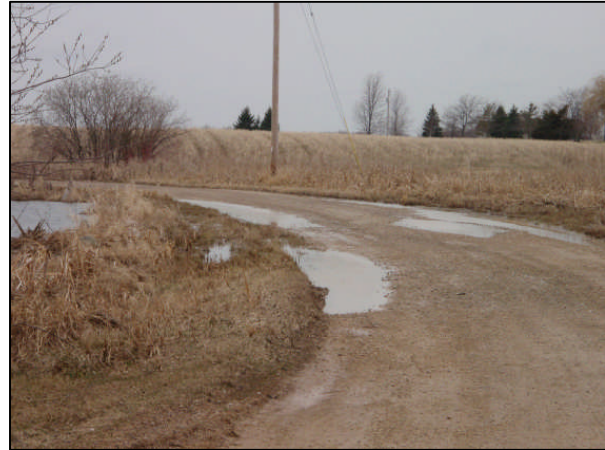
Round Lake Road, beside Round Lake, often gets washed out due to upslope drainage.
