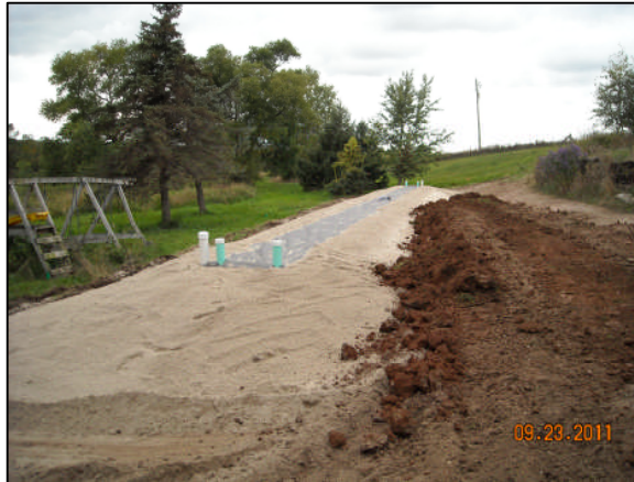
After – A new, fully functioning mound system replaces the old holding tank.
