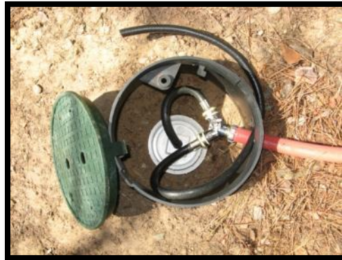
D) Runoff collector and sampler housing
