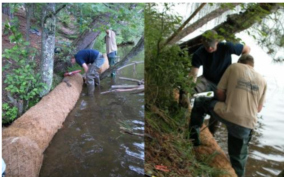
Figure 26 Installation of biologs at BJW-SP property on LSG in June 2011. Biologs were secured to the lake bed using cabled earth anchors and then planted with native wetland plants.
