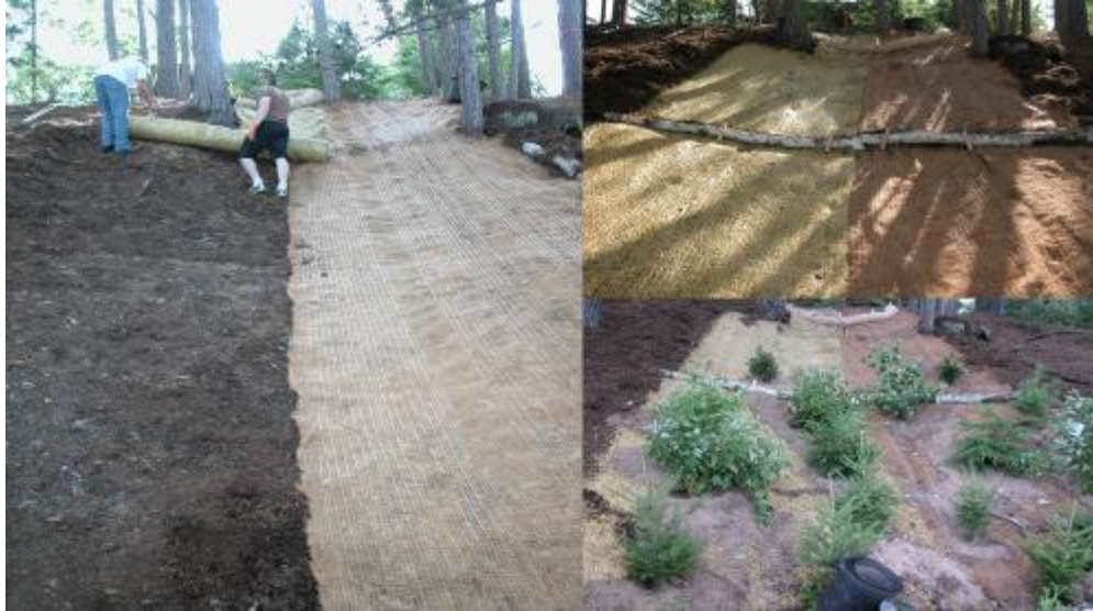
Figure 24 Installation of erosion control blankets in the summer of 2011 on Mirek’s Property, LSG Lake. Two types of blankets were used, coconut coir and straw
