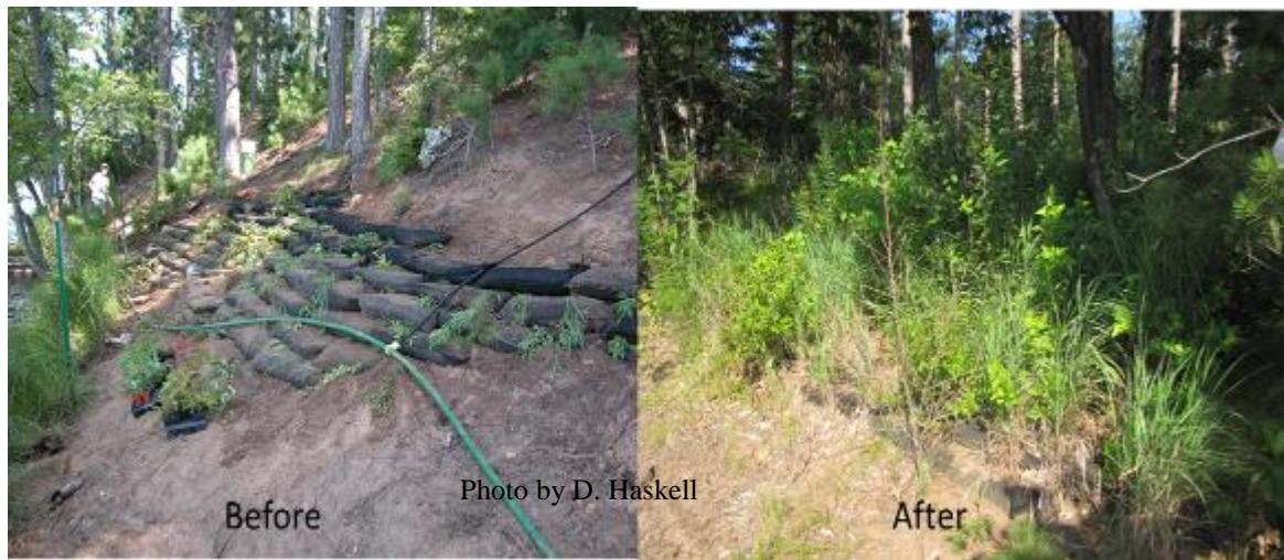
Figure 23 Photos of geotextile bags installed on Lou Mirek's property during the summer of 2011 and 2012.
