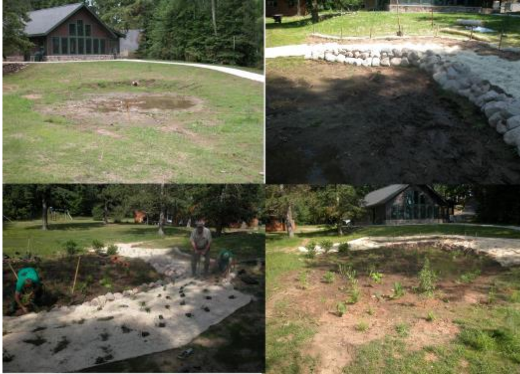
Figure 25 Construction of rain garden on Waldmann’s Sunset Pine property in 2011. Rain garden was designed to retain water runoff from hard surfaces surrounding rental cabins. Native wetland plants were integrated throughout the rain garden.
