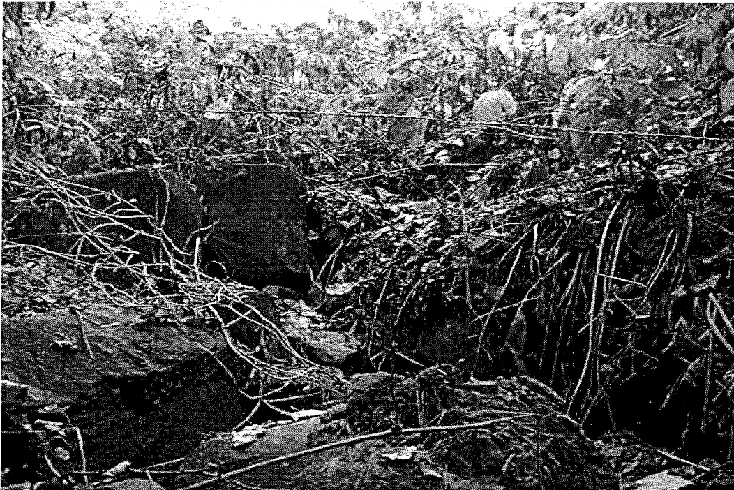
Figure 2. Pikes Bay S. D. effluent discharge pipe, which is covered with large stones.
