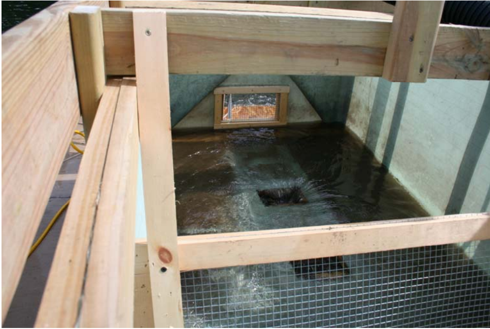
Figure 8. Screened holes added to the HCS catch basin looking from the primary containment area.
