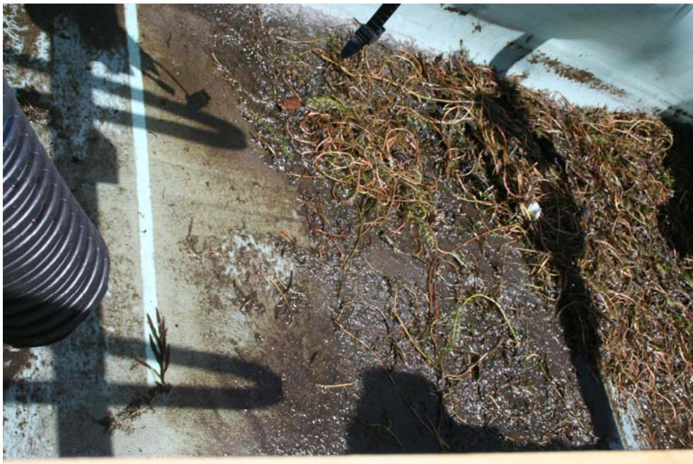
Figure 7. Sediment that was caught in the HCS catch basin.
