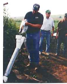
Lee Montgomery, Lovelace Pump Co., pours bentonite chips down a well to properly seal it.
