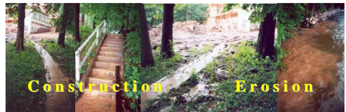
Figure 1 – In violation of erosion control regulations, measures to reduce or prevent erosion have not been installed on this new construction site. On the far right lake water is clouded by sediment that cascaded directly down the landowner's stairway.
