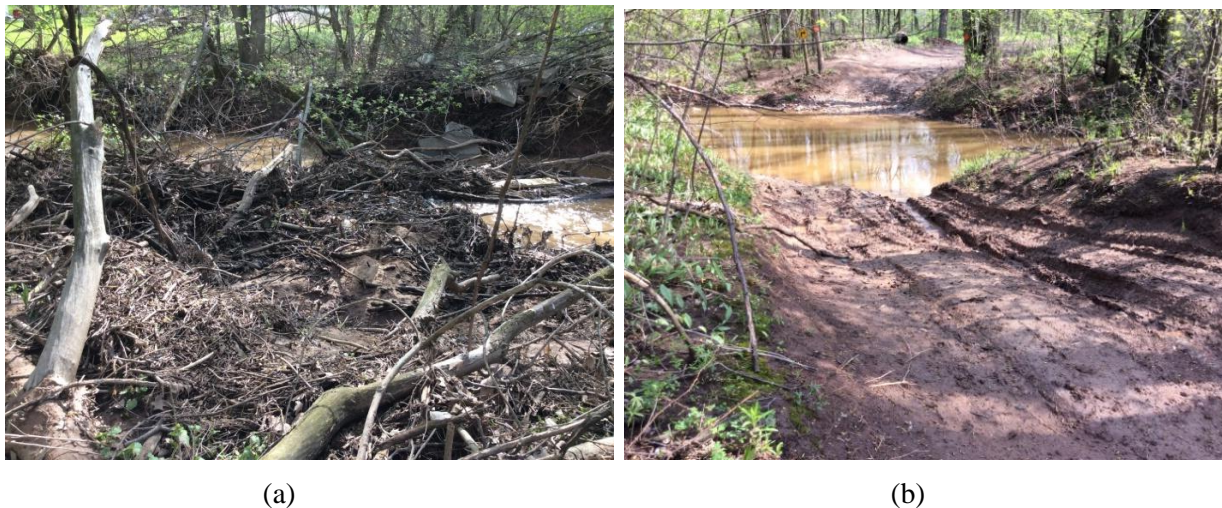
Figure 25. Inventoried sites on Kankapot Creek. (a) Example of large amount of debris blocking flow. (b) Example of crossing that needs to be stabilized.
