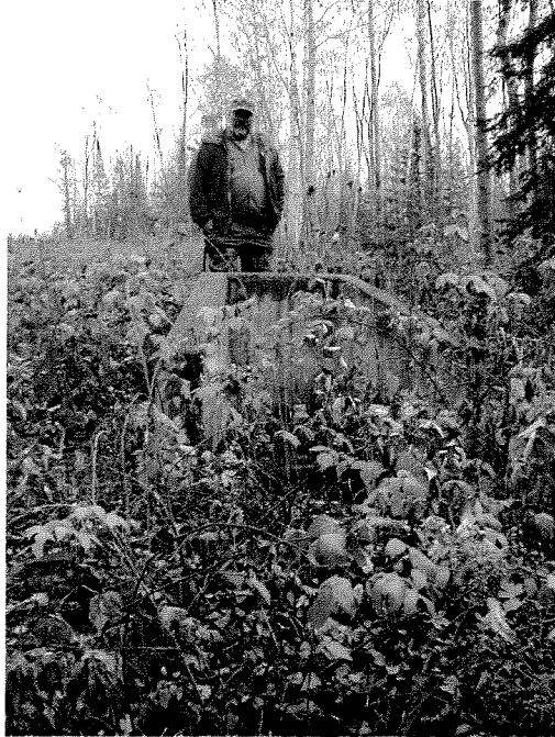
Cornucopia/Bell Sanitary District wastewater discharge outlet - view facing outlet.
