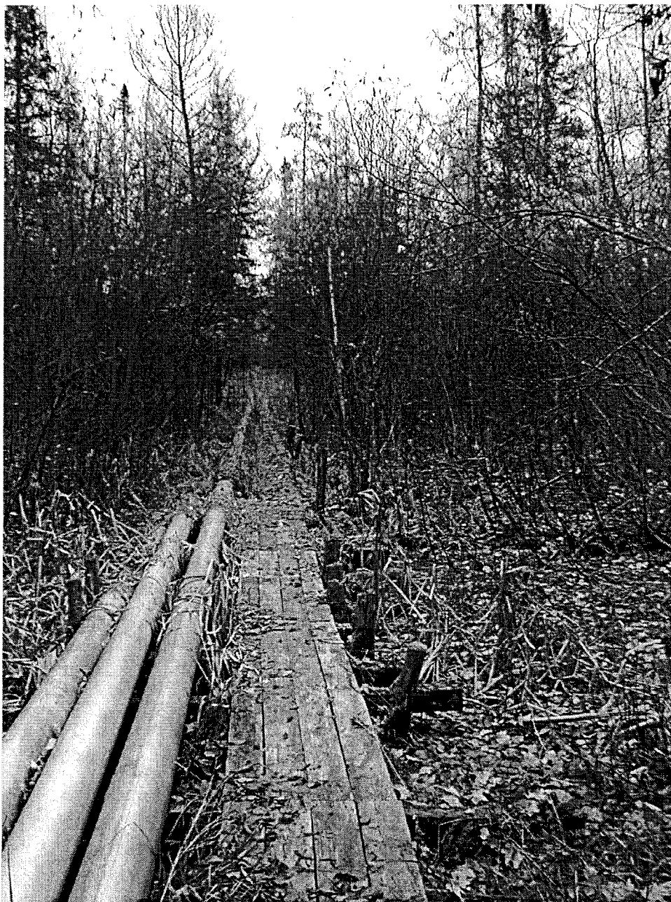
Figure 2. Drummond WWTF outfall pipe into bog.
