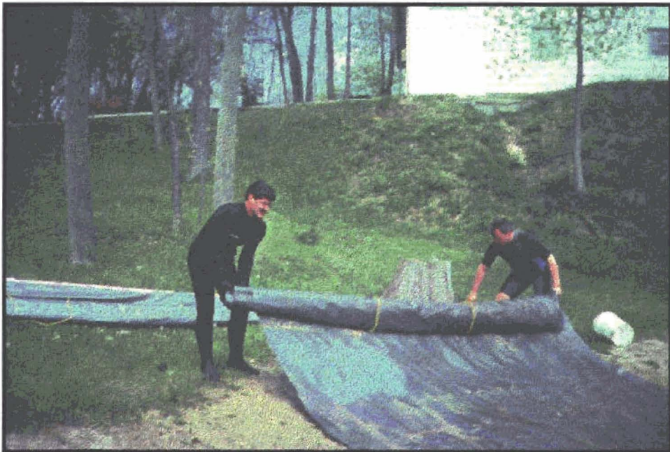
Figure 14 ROLLING UP A ROLL OUT BENTHIC BARRIER AS IT IS PULLED IN AT THE SHORELINE
