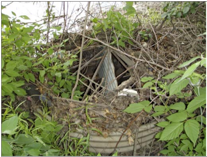
Figure 3.8: Outlet structure in Pond 3, clogged with debris.
