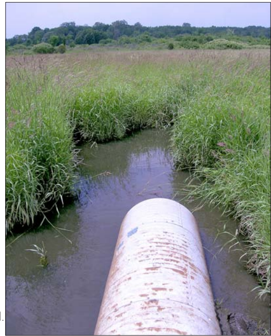
Figure 3.9: Breached berm of Pond 4, looking west from pond.
