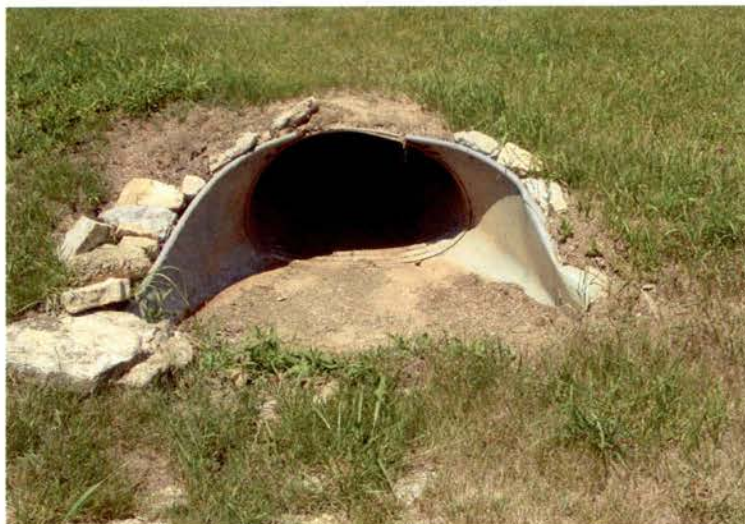
Figure 19. One of four culverts located under Twin Lakes Road, north of Big Twin Lake.
