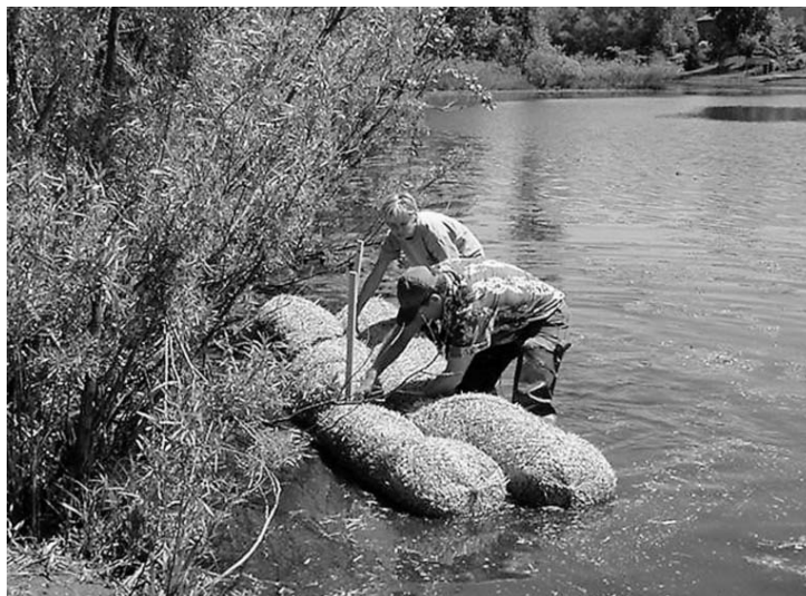
Figure 2.2. Barley straw being installed at South Twin Lake in Burnsville, Minnesota (courtesy of Leslie Yetka, City of Burnsville Natural Resources Department).
