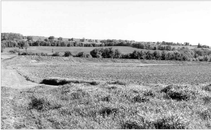
Figure 4.3. A water and sediment control basin being constructed in the Park Lake watershed. An earthen berm (background) and underground outlet were just completed, and the berm had also been seeded (courtesy of Todd Rietmann, Columbia County Land and Water Conservation Department).
