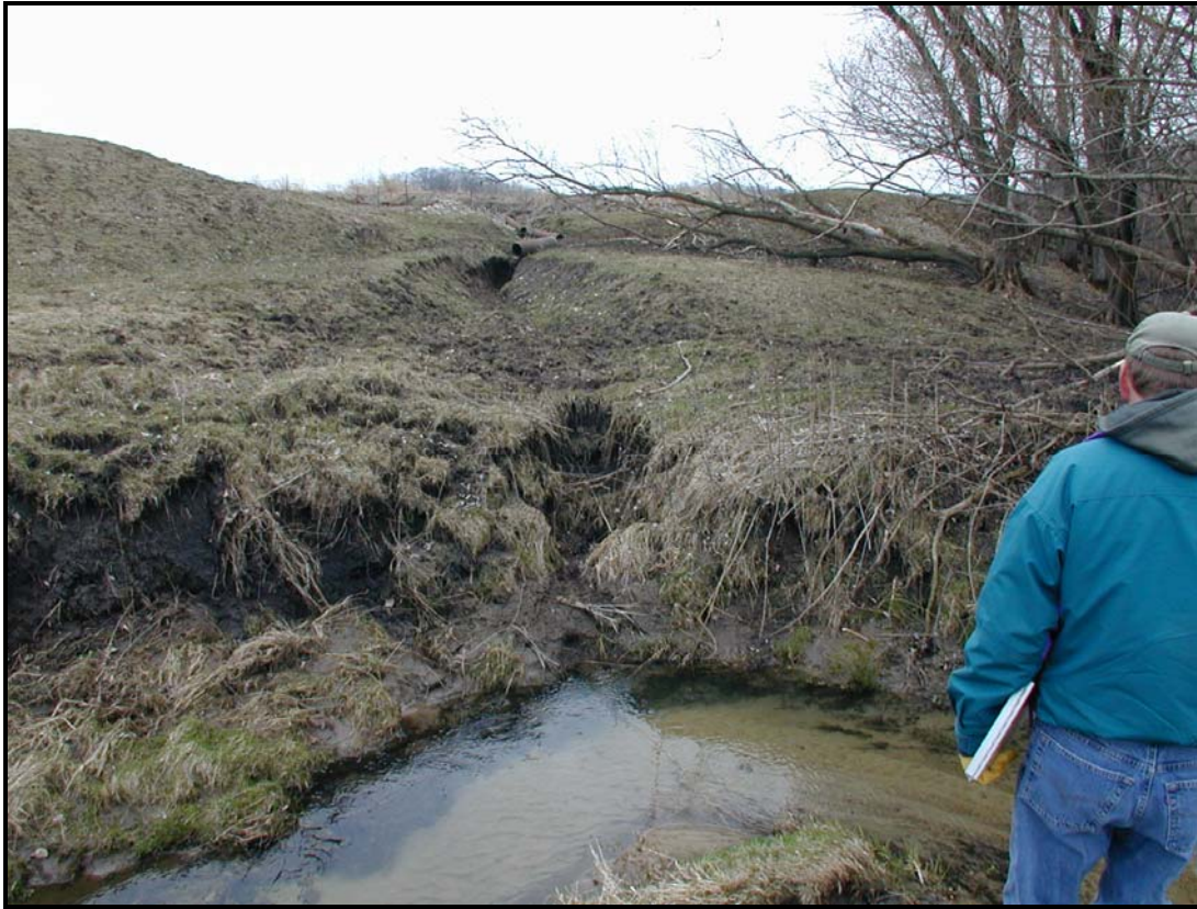
Figure A-6. Stream bank erosion located in middle section of stream.
