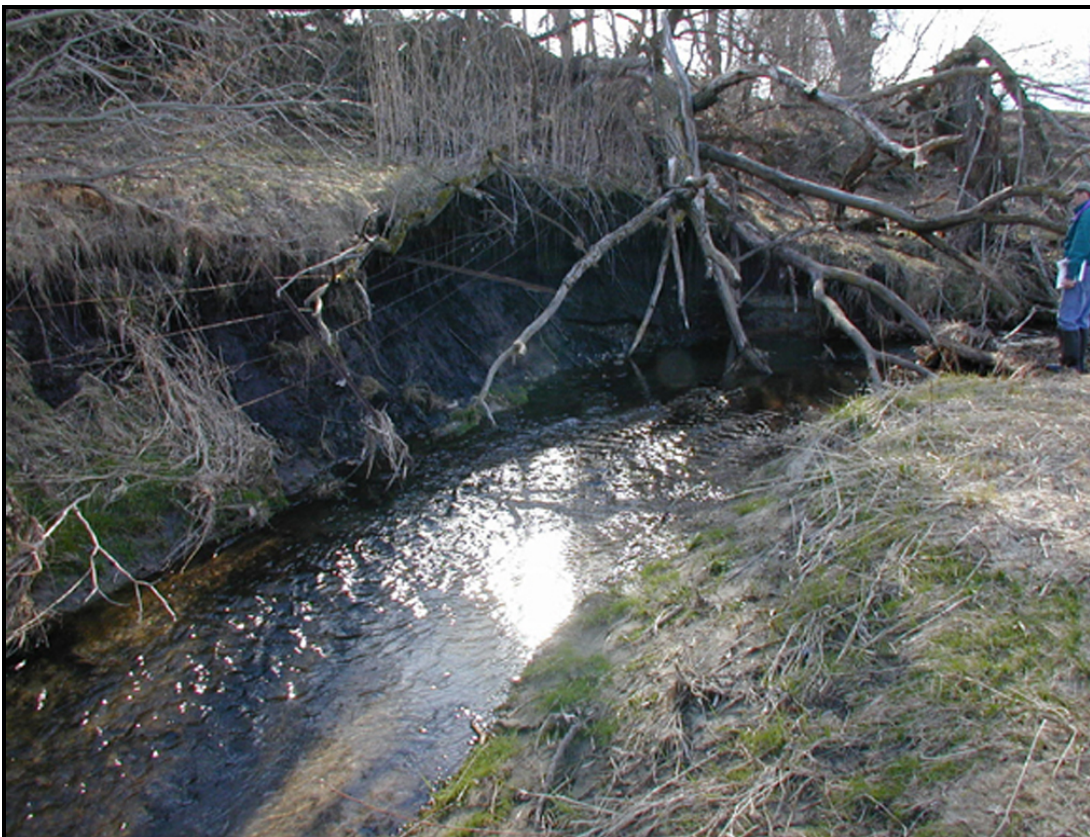
Figure A-5. Stream bank erosion located in upper third of stream.
