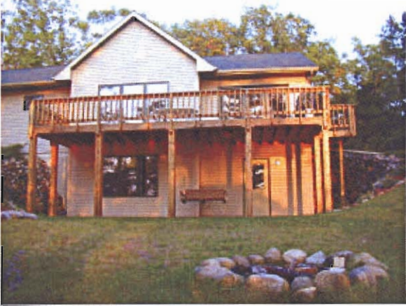
Notice that the metal support beams are covered by wood planks to enhance the visual effect.
