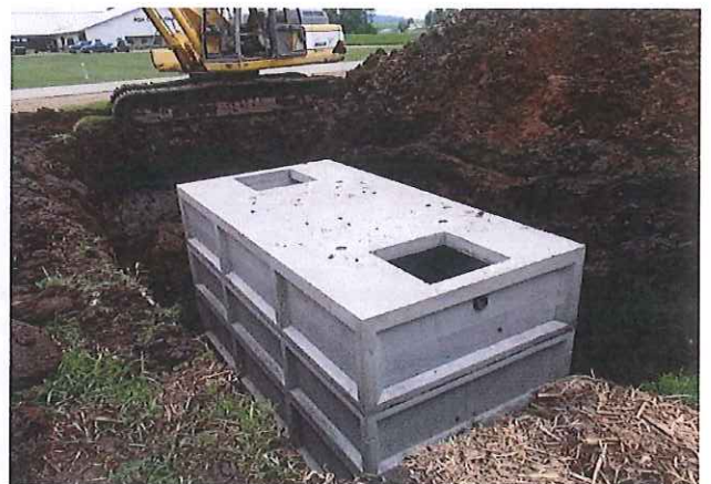
6000 gallon collection tank installed
