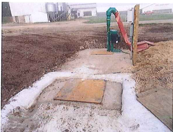
Tank with covers in place
