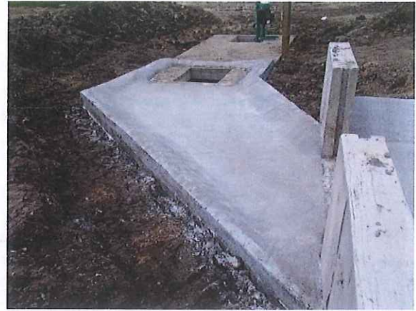
Channel from outlet screen to collection tank
