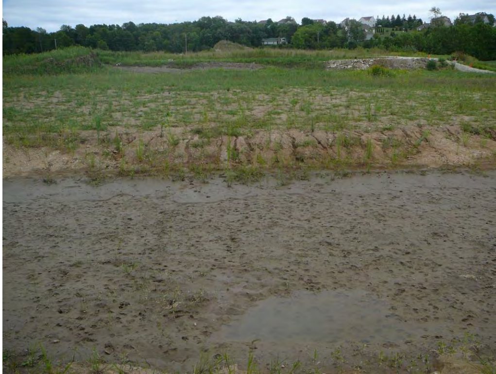
Photo 21. East view of newly created stormwater detention pond in center of project area and fill pile visible in background.
