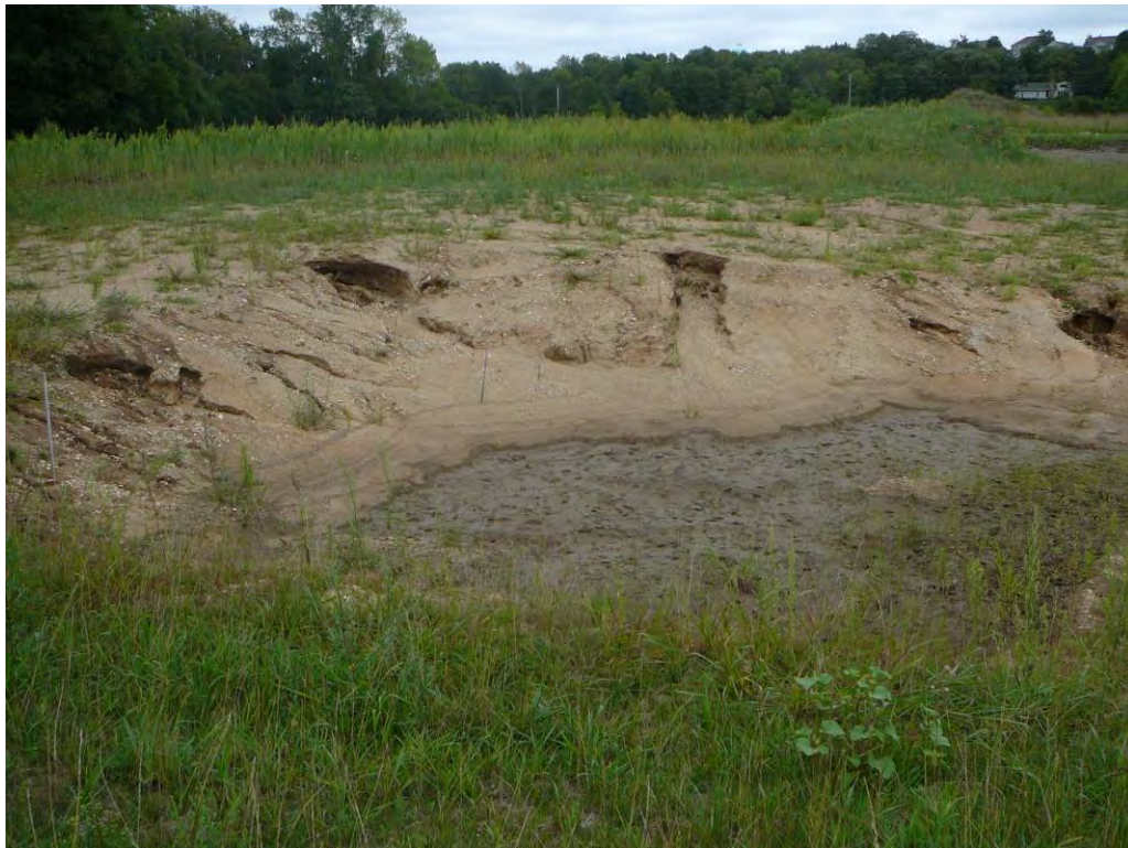
Photo 20. Erosion in newly created stormwater detention pond in center of project area.
