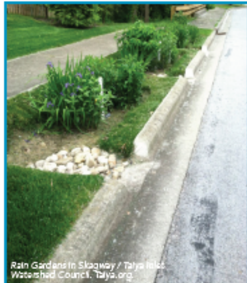
Infiltration basins behind curb cuts
