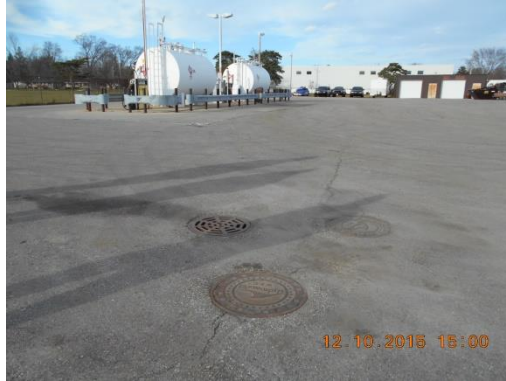
Hydroworks Separator near fueling center.
