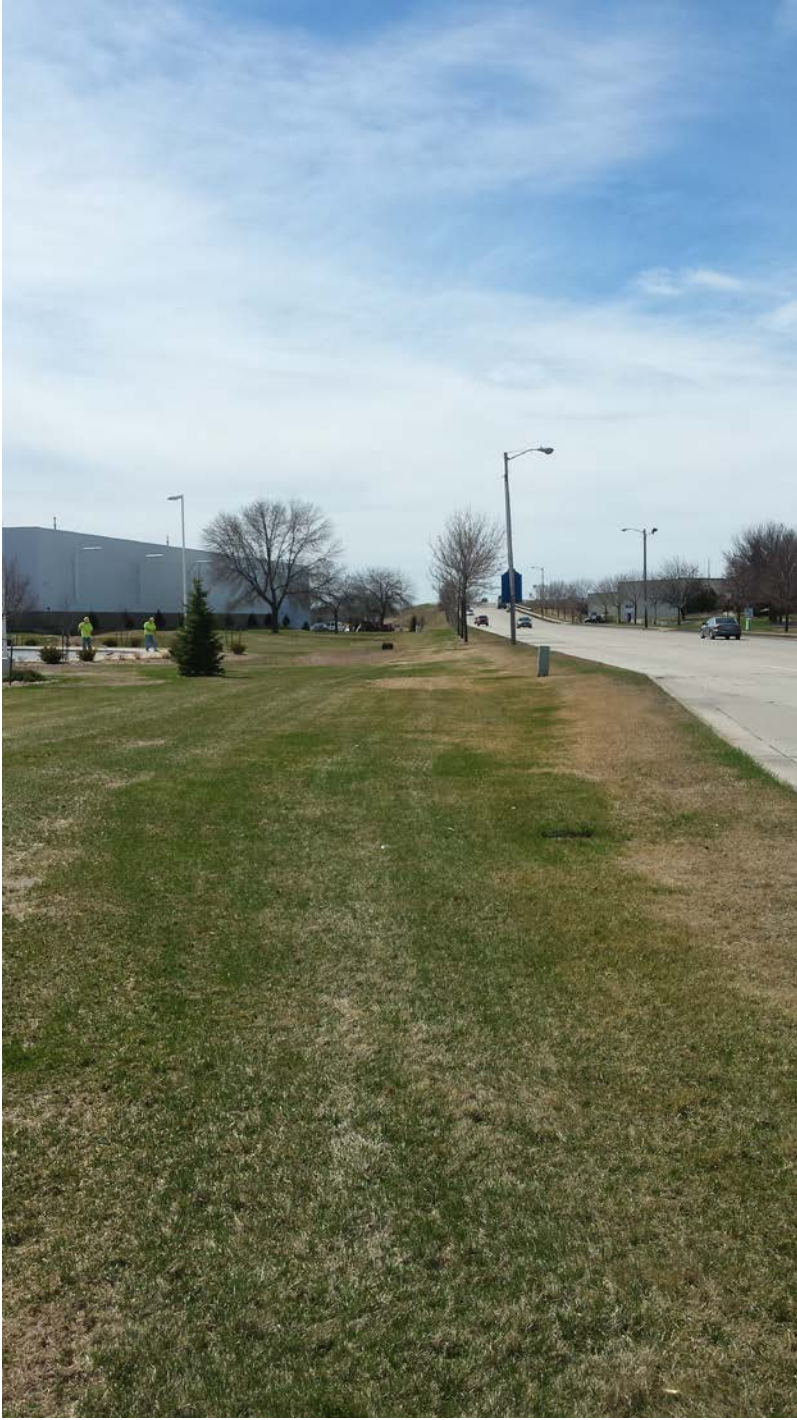
Area of Storm Sewer Installation at Intersection of Industrial Drive and Bell Street Looking West.
