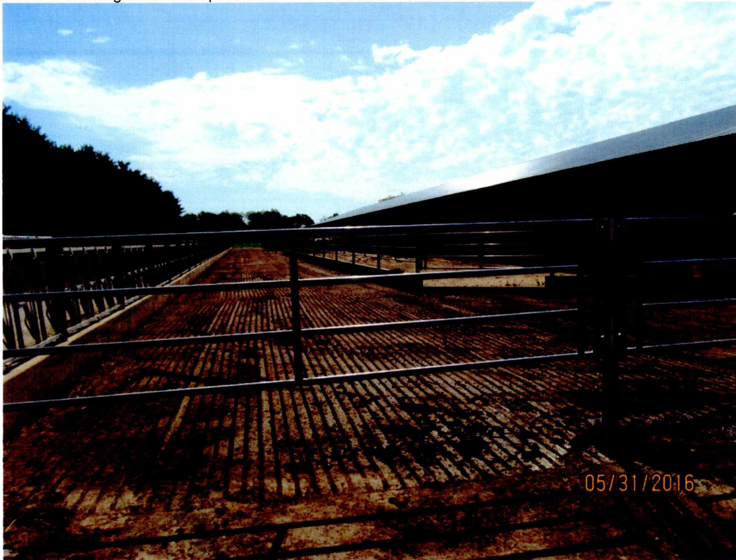
Photo 1: Looking east at completed concrete feed lanes in the former Pen 26 at Gus’ farm.
