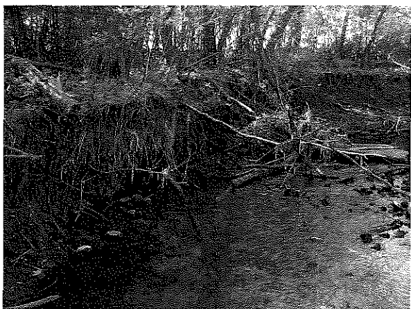
Figure 3.02-9 Severe (Rating 4) Streambank Erosion (or-06, Photo 183)
