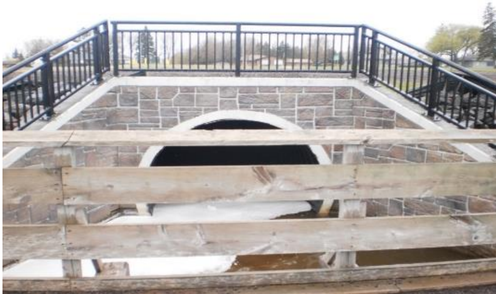
Figure 14. Bridge at Faxon Creek Culvert (BARK-ST) where Routine Samples were Collected Twice Weekly and During Rain Events.
