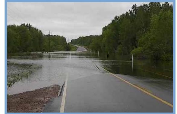
Figure 24: Flooding of County HWY M in the South Fork of the Eau Claire River Watershed.
