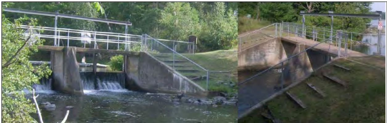
Figure 28 - Mooney Dam (Lower Eau Claire Lake dam) observed during August 2009. Photo during a period of substantial drought, and provides insight into low-flow conditions.
