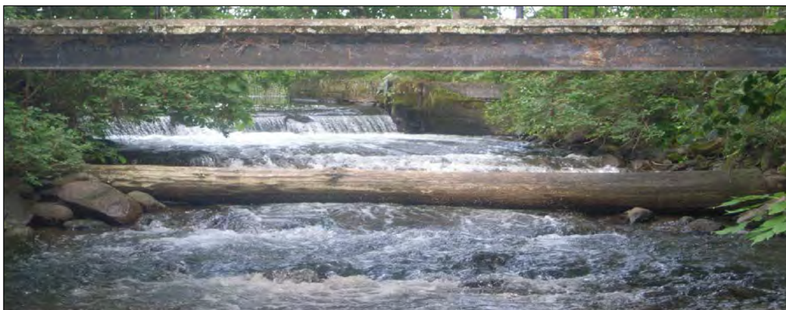
Figure 32 - Upper Eau Claire Lake dam observed during August 2009. This observation was made during a period of substantial drought, and provides insight into low-flow conditions.
