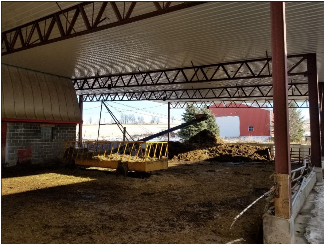
After: Roofed feedlot and manure stack
